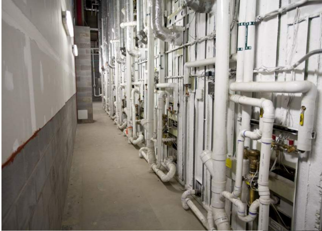
Allegan County Jail – Rear Mechanical/Plumbing Chase
